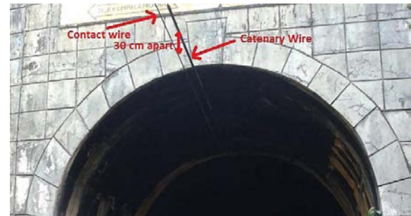
Fig. 17. Uninsulated traction conductor drawn very close to the earth potential surface.
